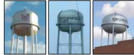
Illustration 10-1 Elevated Storage Tanks
